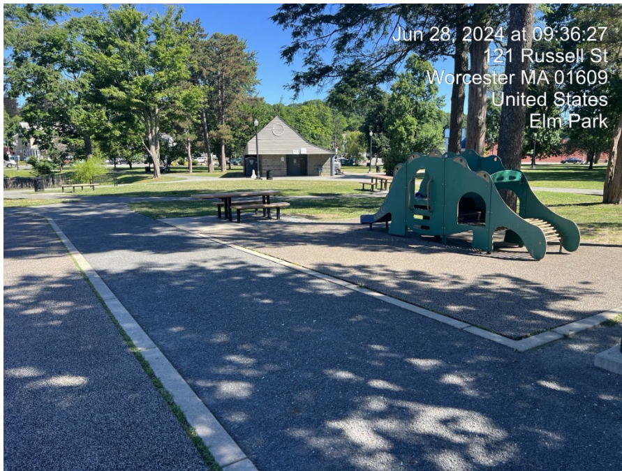
Area E - proposed removal of existing bituminous asphalt walkway between playground equipment Area A and E and replace with PIP. Typical at four locations.
